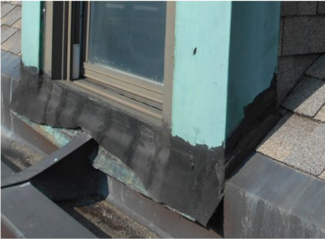
Flashing repairs needed around courthouse windows.
