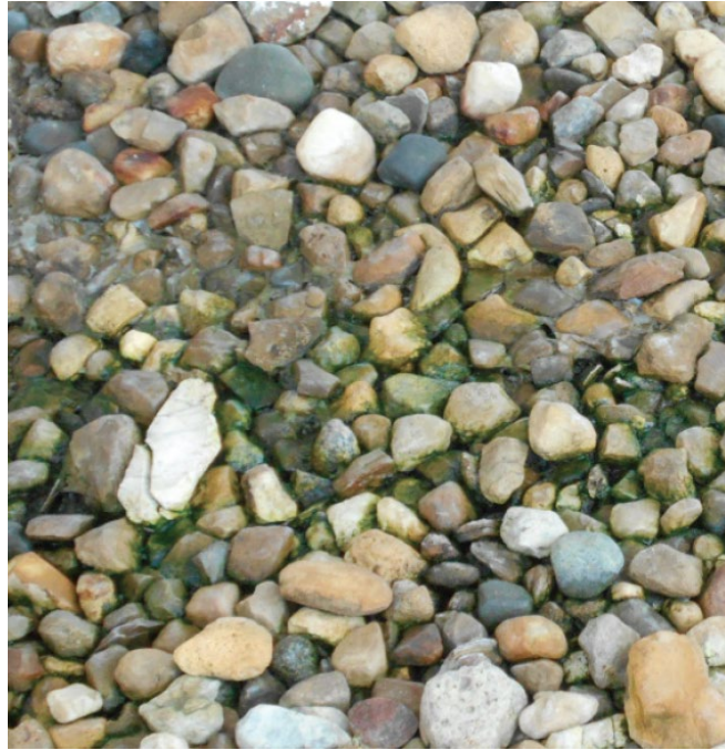
Standing water, moss, and plants growing in Courthouse Annex roof.
