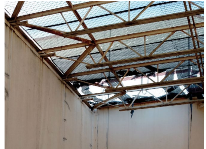
Damage in lightwell at Satellite Corrections facility.
