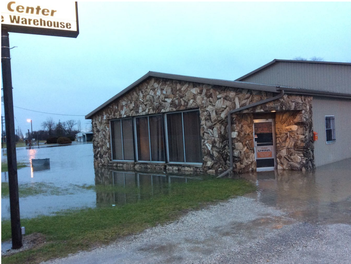
This is Corky's Auto center on Rt. 45 in the background is the entrance to Fountain Valley trailer park, at times the water is in the building a foot or more deep when the culvert has some debris in it and we have a lot of rain.
