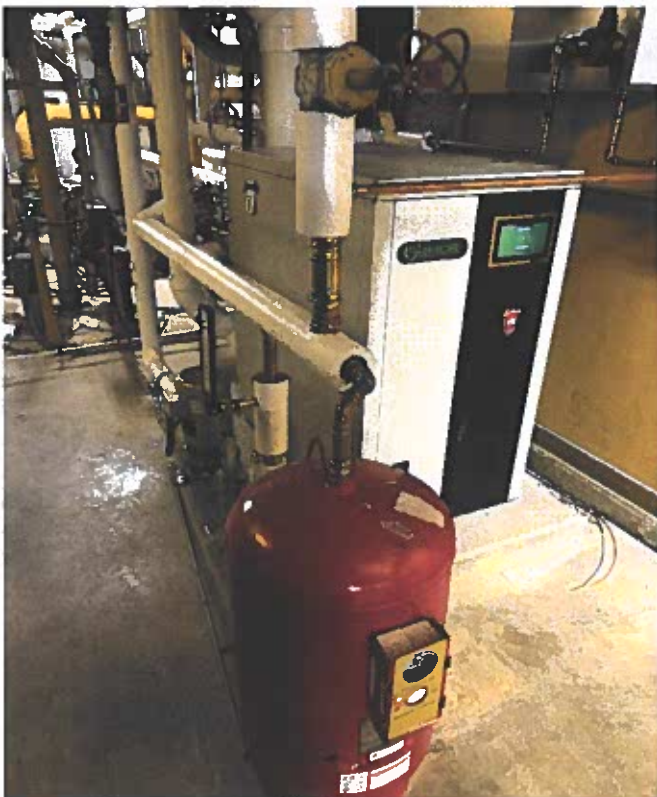
New domestic hot water system
