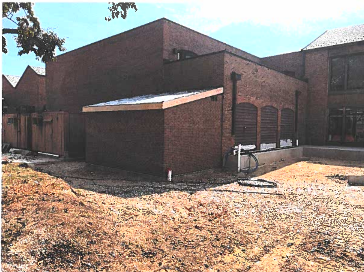
New water feature control and mechanical room
