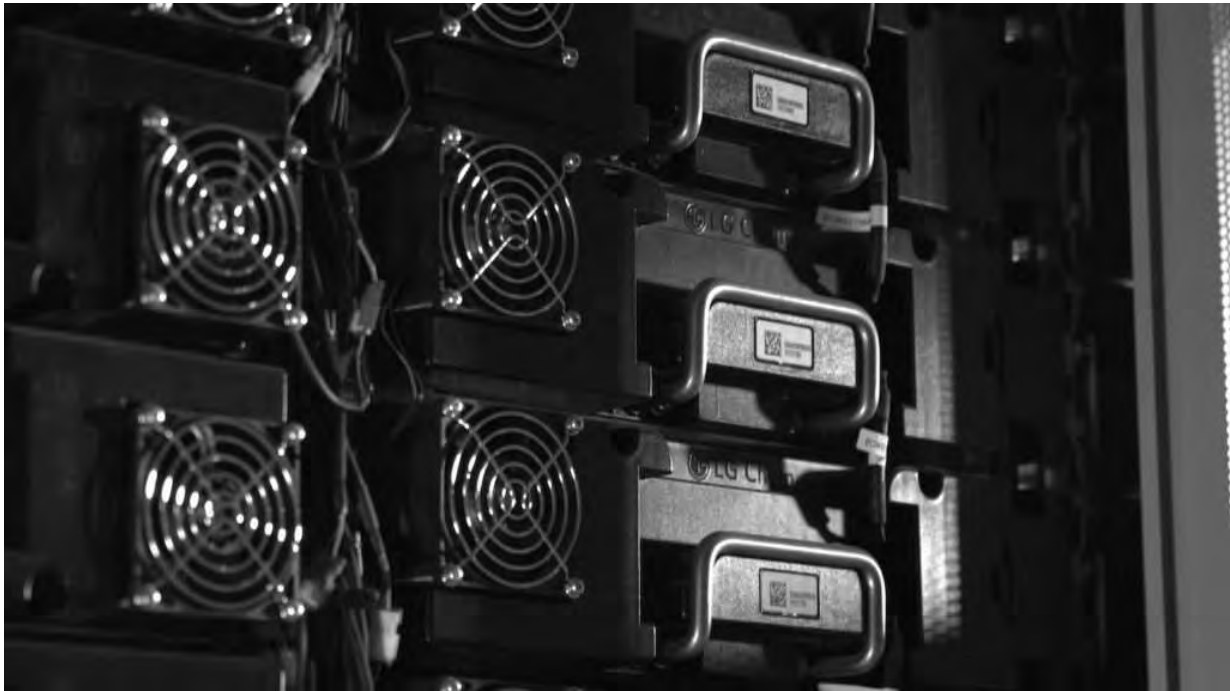
Closeup of battery modules at Moss Landing Energy Storage Facility. Image: Vistra Energy.
