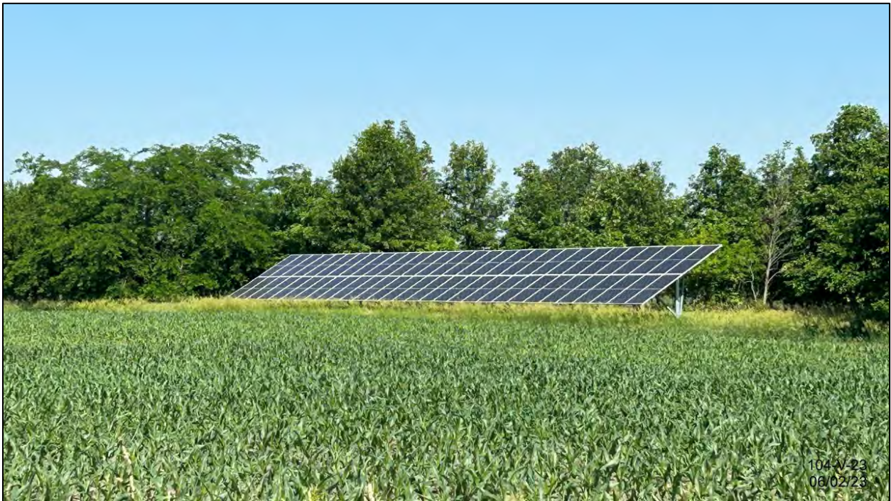
From CR 700E facing NW to solar array
