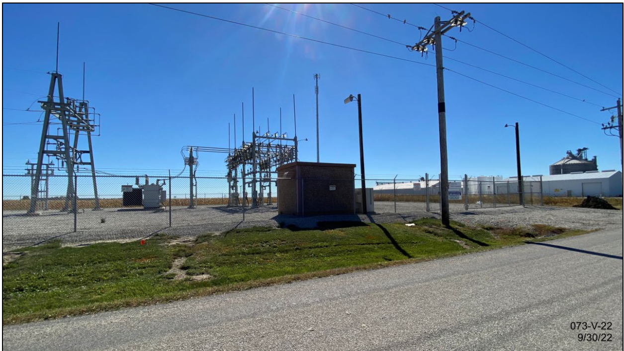
From 700N adjacent to subject property, facing SW to existing substation, monopole, and control building (small structure near road). Premier Co-op is pictured towards the West.
