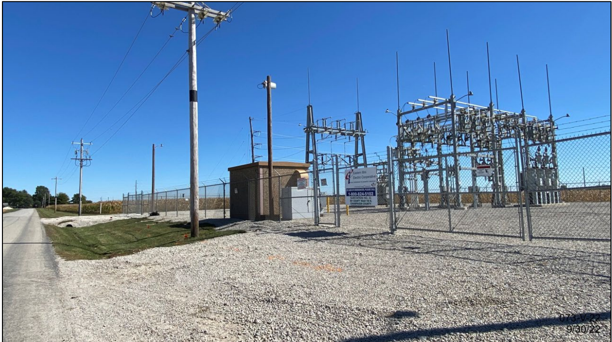
From CR 700N adjacent to subject property, facing SE to existing substation and control building
