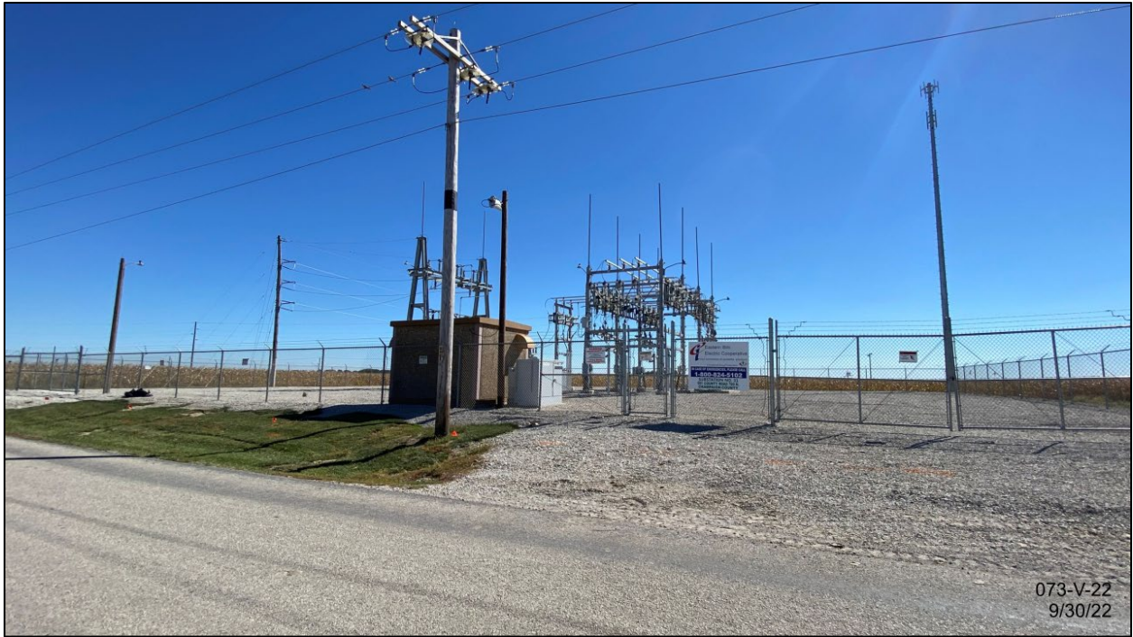
From CR 700N adjacent to subject property, facing SE to existing substation, monopole, and control building
