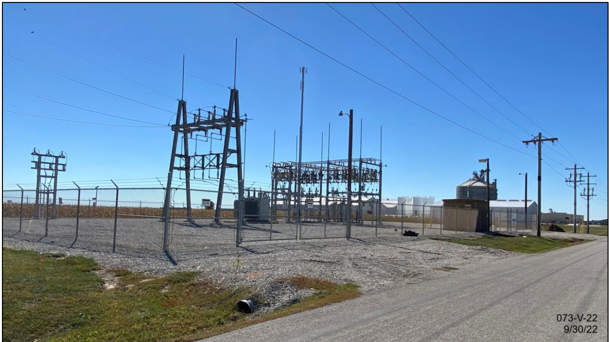
From CR 700N adjacent to subject property, facing SW to existing substation, monopole, and control building (small structure near road) Premier Co-op is pictured towards the west.
