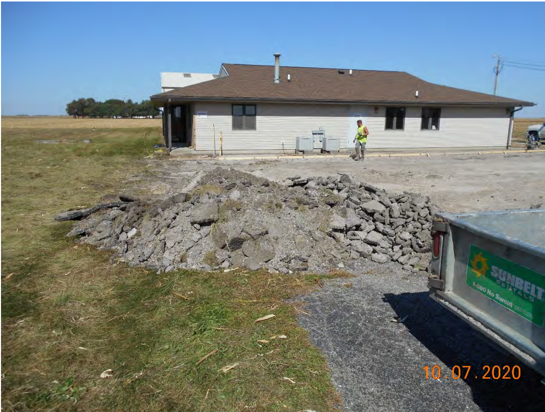
Picture1504- Pile of asphalt you seen in 1501 with trailer pulled up to it.
