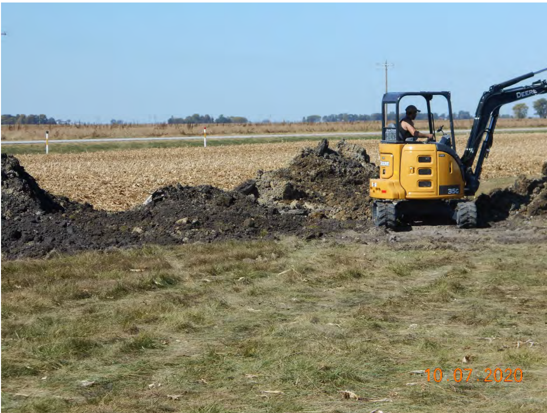
Picture 1503- The hole is covered up. You can see damaged septic pipe. You can also see pieces of asphalt on top of ground.
