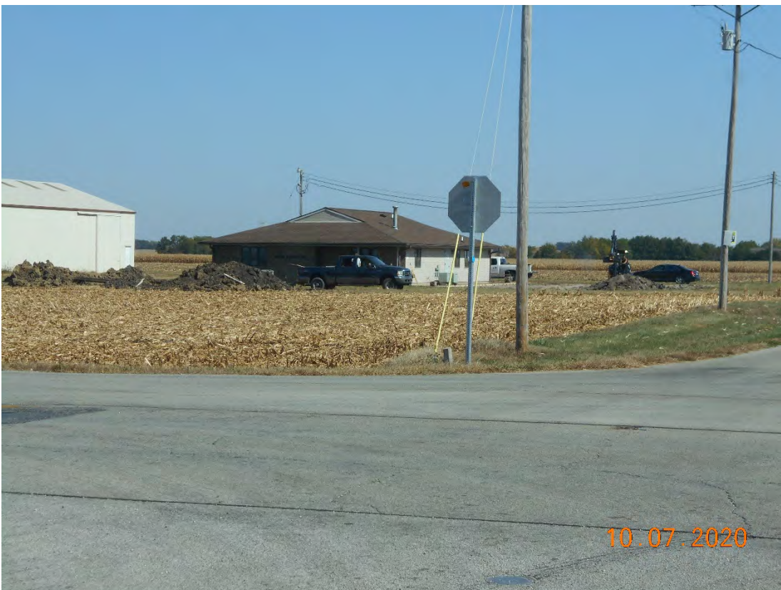
Picture 1501- Trailer is in different spot. You can see pile of asphalt and septic field damaged pipe.
