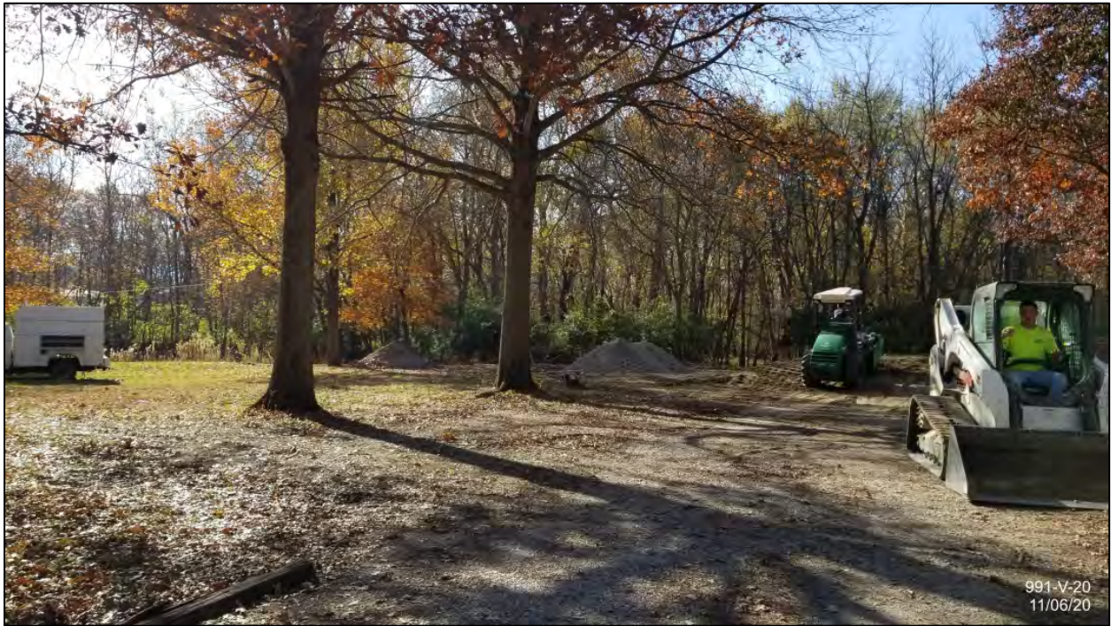
From driveway facing west to clearing south of shed (shed is off to the right)
