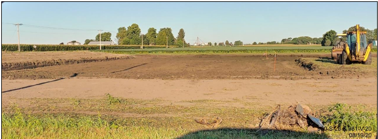
From CR 2000E facing West, large dirt pile to right of backhoe (see next photo)
