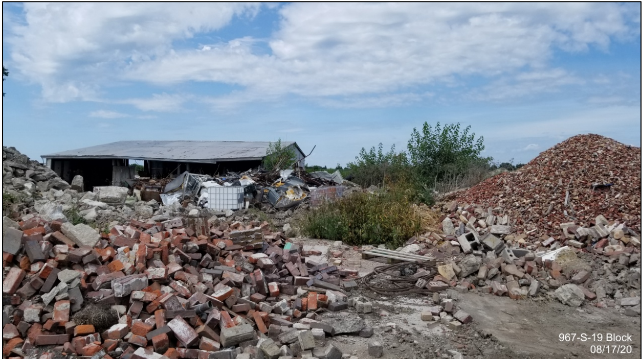
Between storage shed and existing building – materials to be crushed and demolition debris
