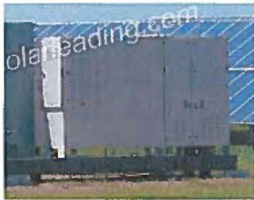
5. Power Plant Controller
