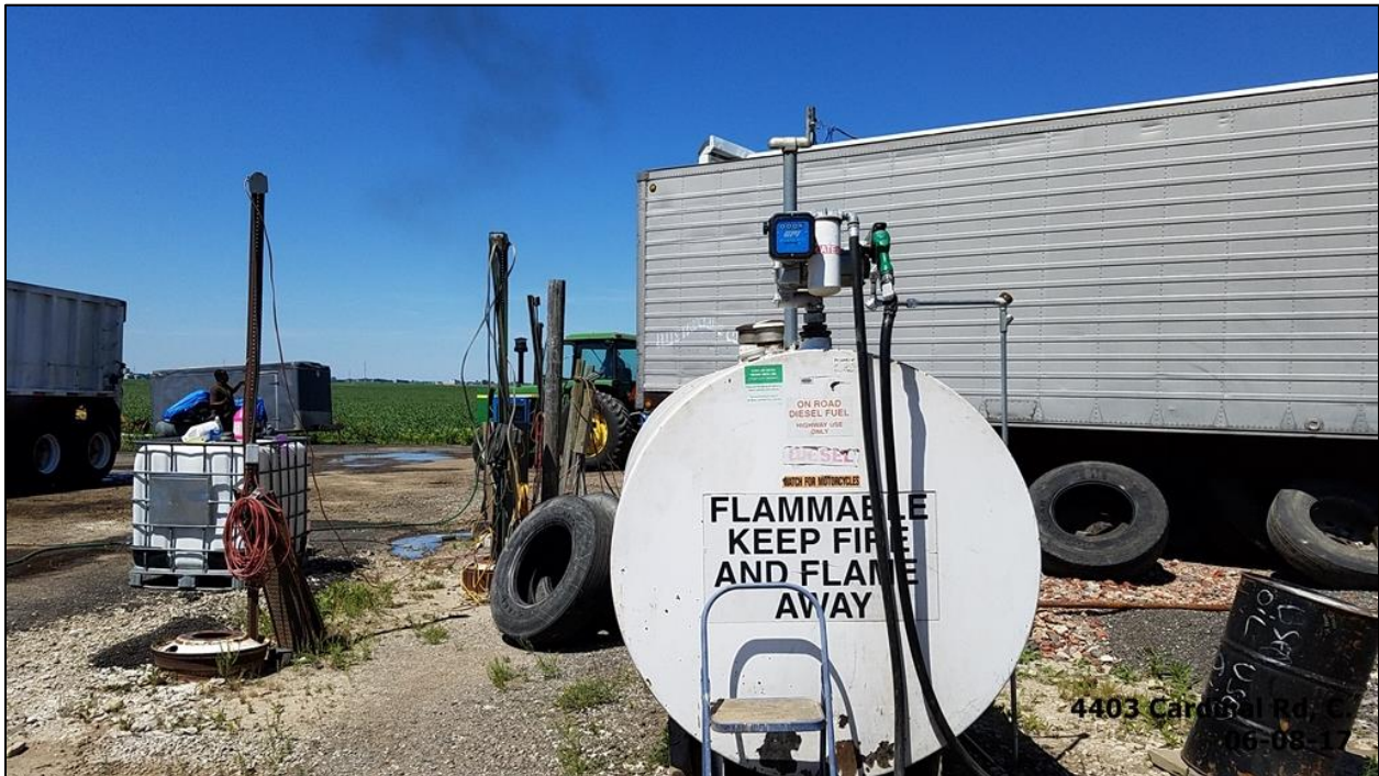
Diesel fuel above ground tank, south of large shed
