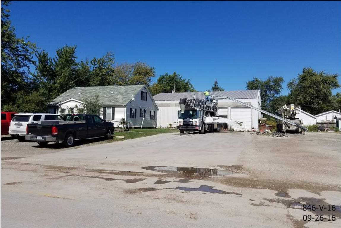
Existing guest house and storage building – addition will be to right of storage building
