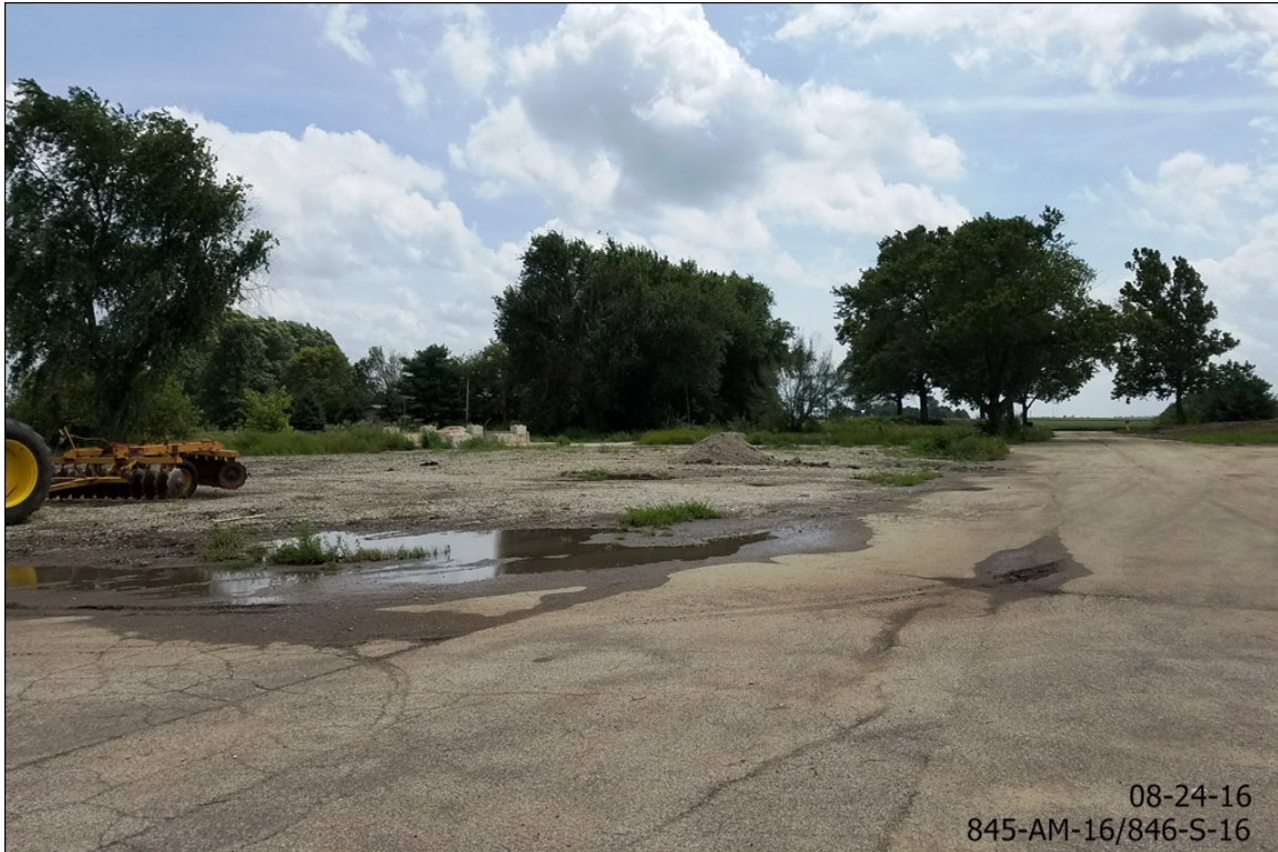
Proposed Truck Terminal shop space, from north end of property facing southeast
