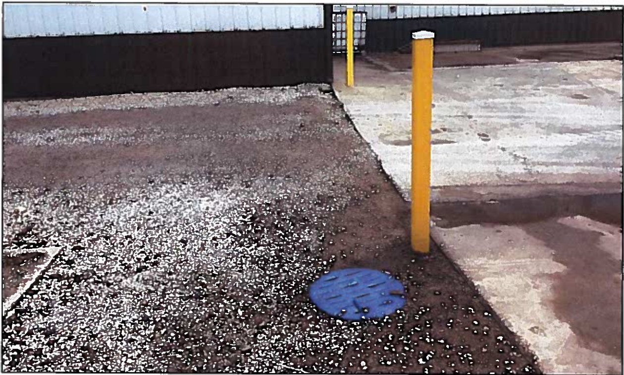
Catch basin by load out area
