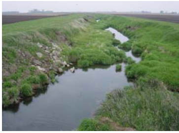
April 2005: Small "floodplain" formed from prior bank failures.
