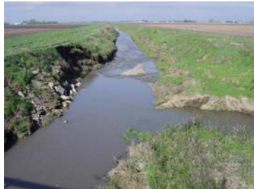
April 2006: Bank failure following spring rain.
