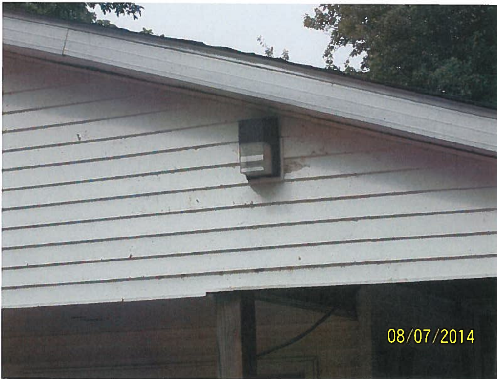
Exterior lighting on Business building
