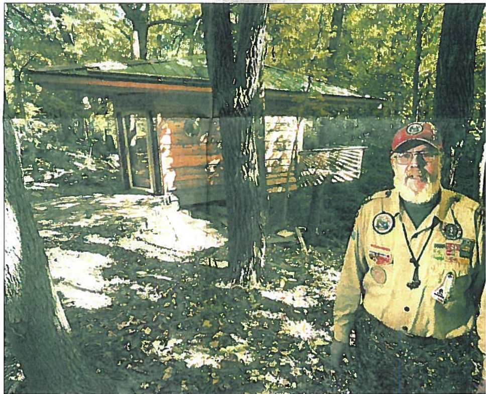
Above: Scout leader Denny Anderson talks about the Green 17, which he designed at Camp Drake near Oakwood as a self-contained lab with a solar electrical system, super insulation and other amenities. Below: The wires and batteries of the 12-volt electrical system
