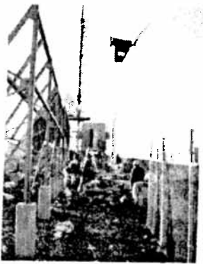
Proven Energy 6kW turbine powering telecommunications equipment
