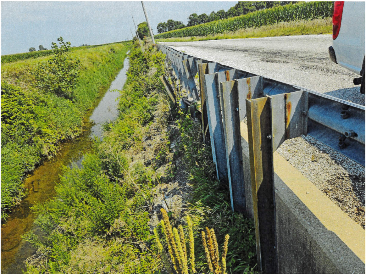
Photo 1: Slide correction area along CR 975 E (looking north)
