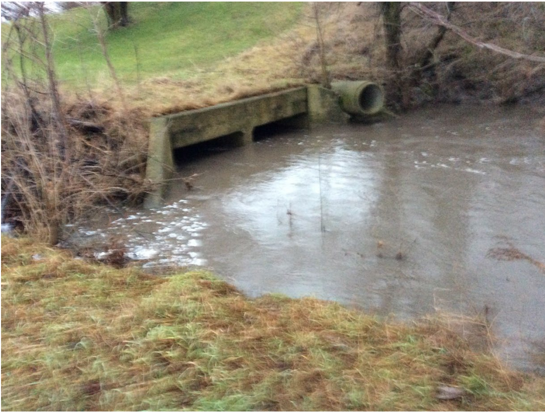
This is the West end of the culvert during a normal rain.
