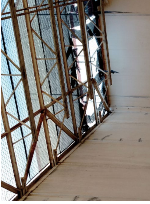
Damage in lightwell at Satellite Corrections facility.
