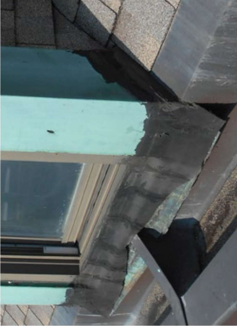
Flashing repairs needed around courthouse windows.
