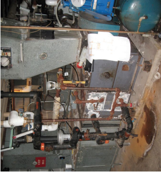
Nursing home return air handlers require replacement.
