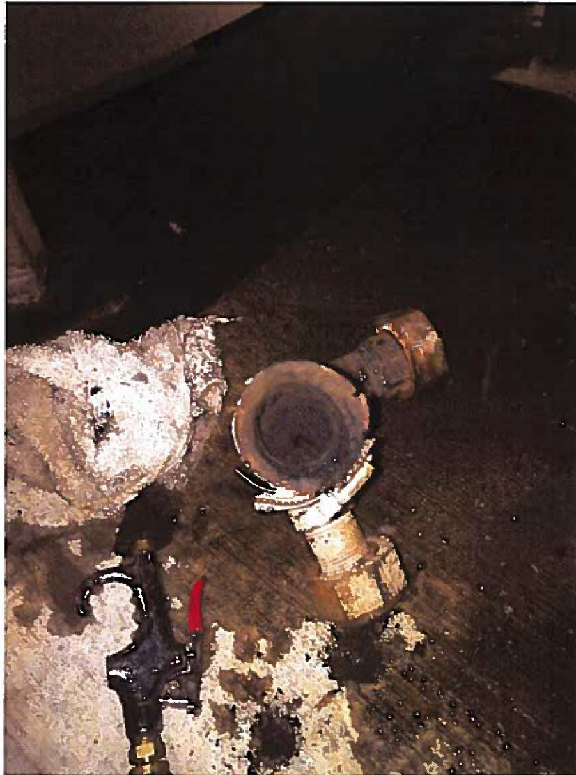
Condensate drains plugged with scale and carbon build up.
