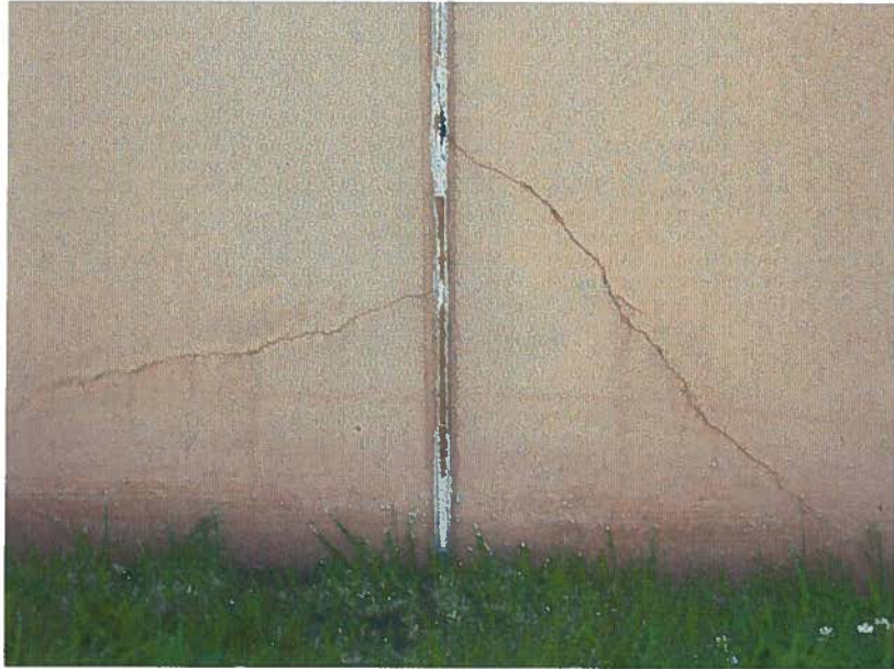
Figure 9 - Cracks at panel corners; and breach in joint sealant (Brenner photo)
