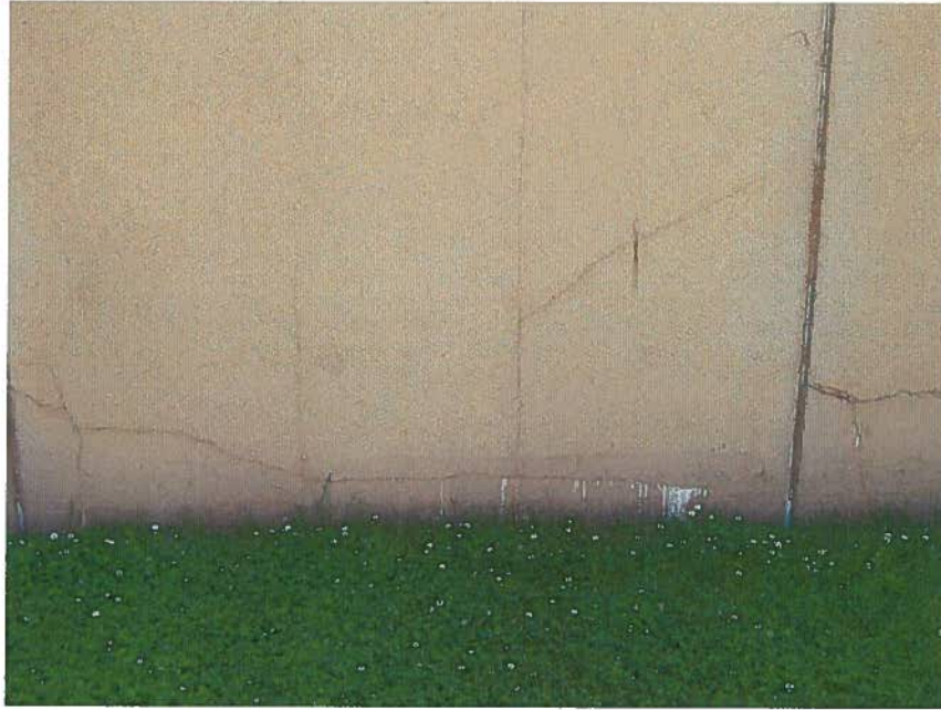
Figure 11 - Various types of cracking in a wall panel, and efflorescence (Brenner photo)
