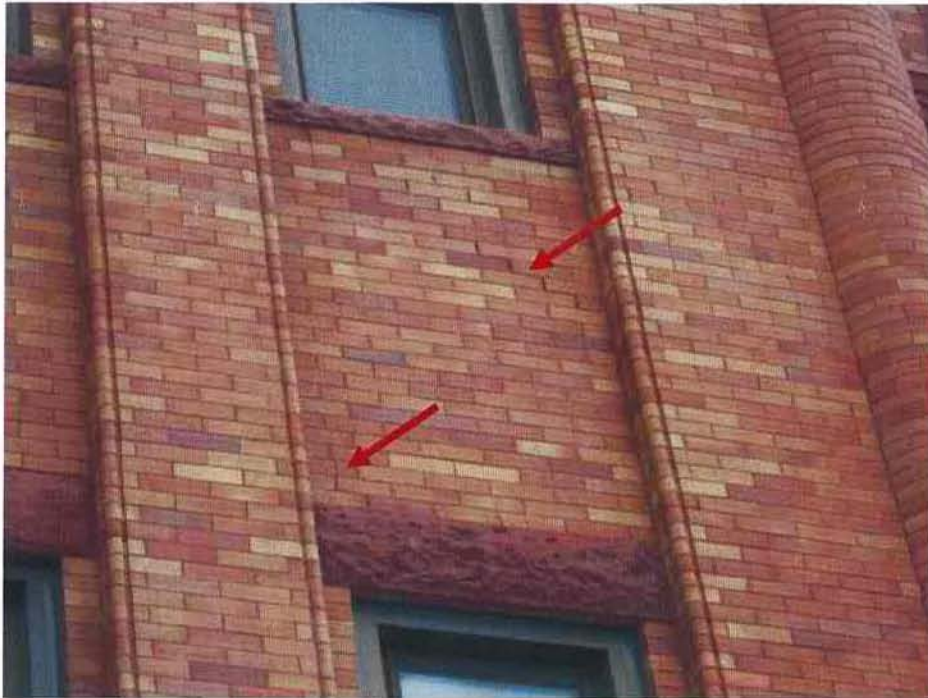
Photo No. 1: West façade spandrel area – typical area of step cracking with cracked brick and open mortar joints.
