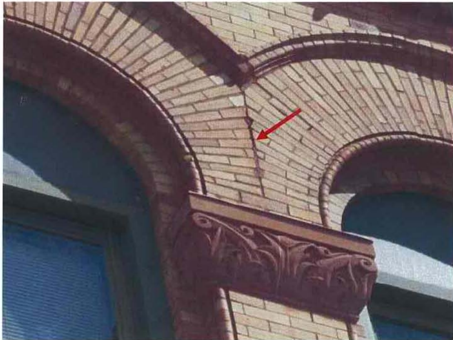
Photo No. 3: West façade third floor arched window head – open joints at brick masonry.
