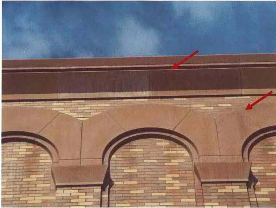
Photo No. 3: North façade cast stone cornice – staining.
