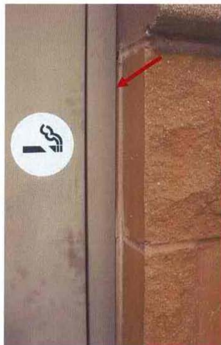
Photo No. 5: North façade grade level exit door – no sealant in joint between door frame and cast stone building base.
