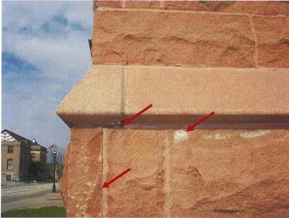
Photo No. 1: North façade cast stone base and horizontal band – minor cracked and open mortar joints and efflorescence. Note: Cast stone was used on the new addition to simulate cut natural stone.
