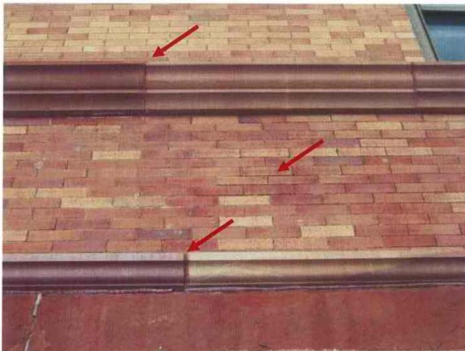
Photo No. 2: South façade brick spandrel and sandstone horizontal bands – typical area of open mortar joints at brick spandrel areas and occasionally cracked and open mortar joints at sandstone bands.
